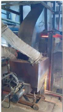
Mobile gas duct of the VER utilization system, with control and measuring devices.
